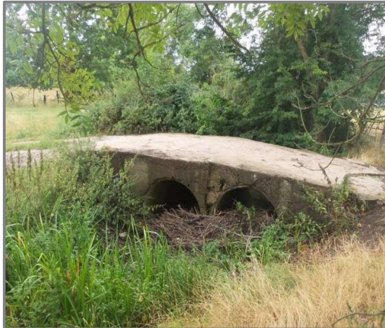
Bridge blocked by debris
